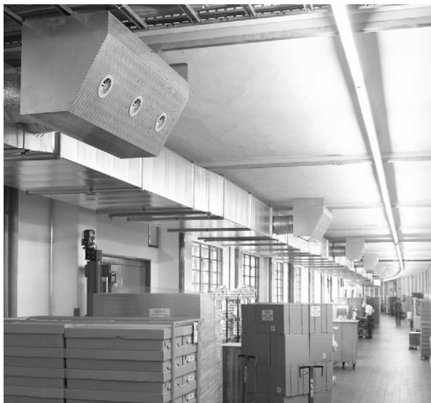
Figure 9: Semi-trapezoidal displacement outlet of size 500 in a production facility
