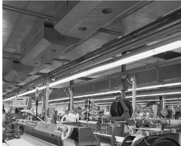
Figure 5: Trapezoidal displacement outlets below the supply air duct in a weaving mill
