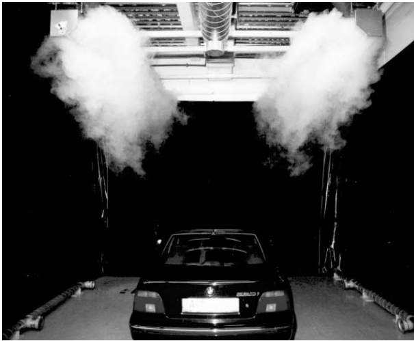
Figure 4: Semi-trapezoidal displacement outlet in a test room of the automotive industry
